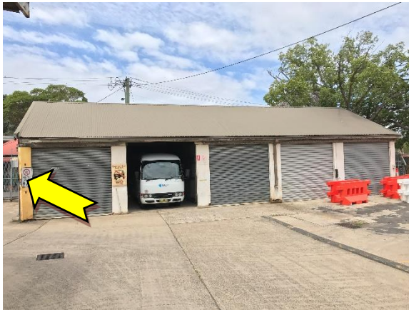
Photo 3. Exterior, throughout, walls – suspected lead-containing yellow upper paint system.
