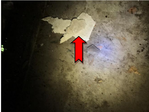
Photo 1. Interior, ground level, west room, debris – asbestos-containing fibre cement sheeting.
