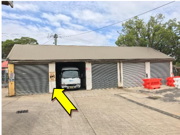
Photo 4. Exterior, north elevation, wall – suspected lead-containing white upper paint system.
