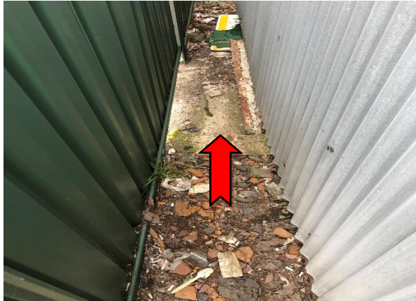
Photo 2. Exterior, throughout, debris – asbestos-containing fibre cement sheeting.
