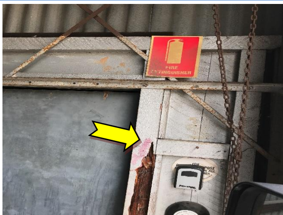
Photo 5. Interior, centre room, door frame – suspected lead-containing white upper paint system.
